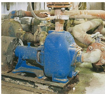
80 Series® pump transferring chemical wastewater to a treatment tank in the Netherlands.
