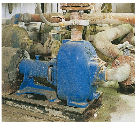
80 Series® pump transferring chemical wastewater to a treatment tank in the Netherlands.
